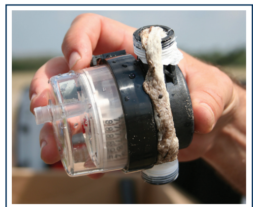
Figure 6. Filamentous sulfur slime completely clogging a small water meter.
